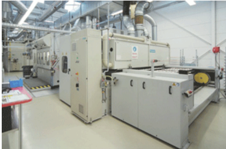
Fig.2. Photo Plasmatreat The Openair plasma system (3rd unit from the front) takes up only one meter of a painting line with an overall length of 25m.
